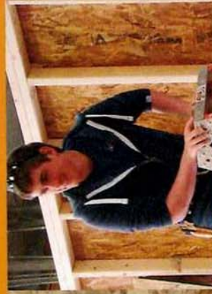
Wesley Brown is going up the ladder to help hold up the sides of the building.
